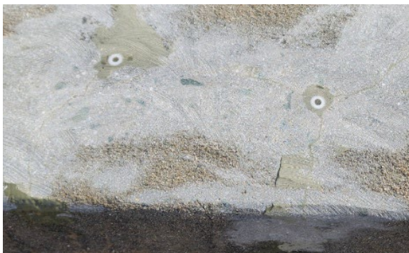
IMPROPER DRILLED-IN PORTS
